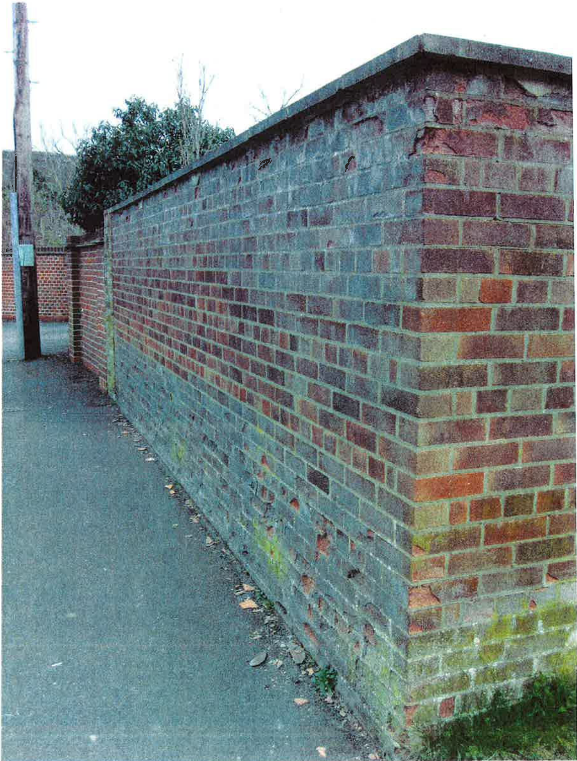
Crumbling bricks in courtyard wall at No 78 Lower Rd.
