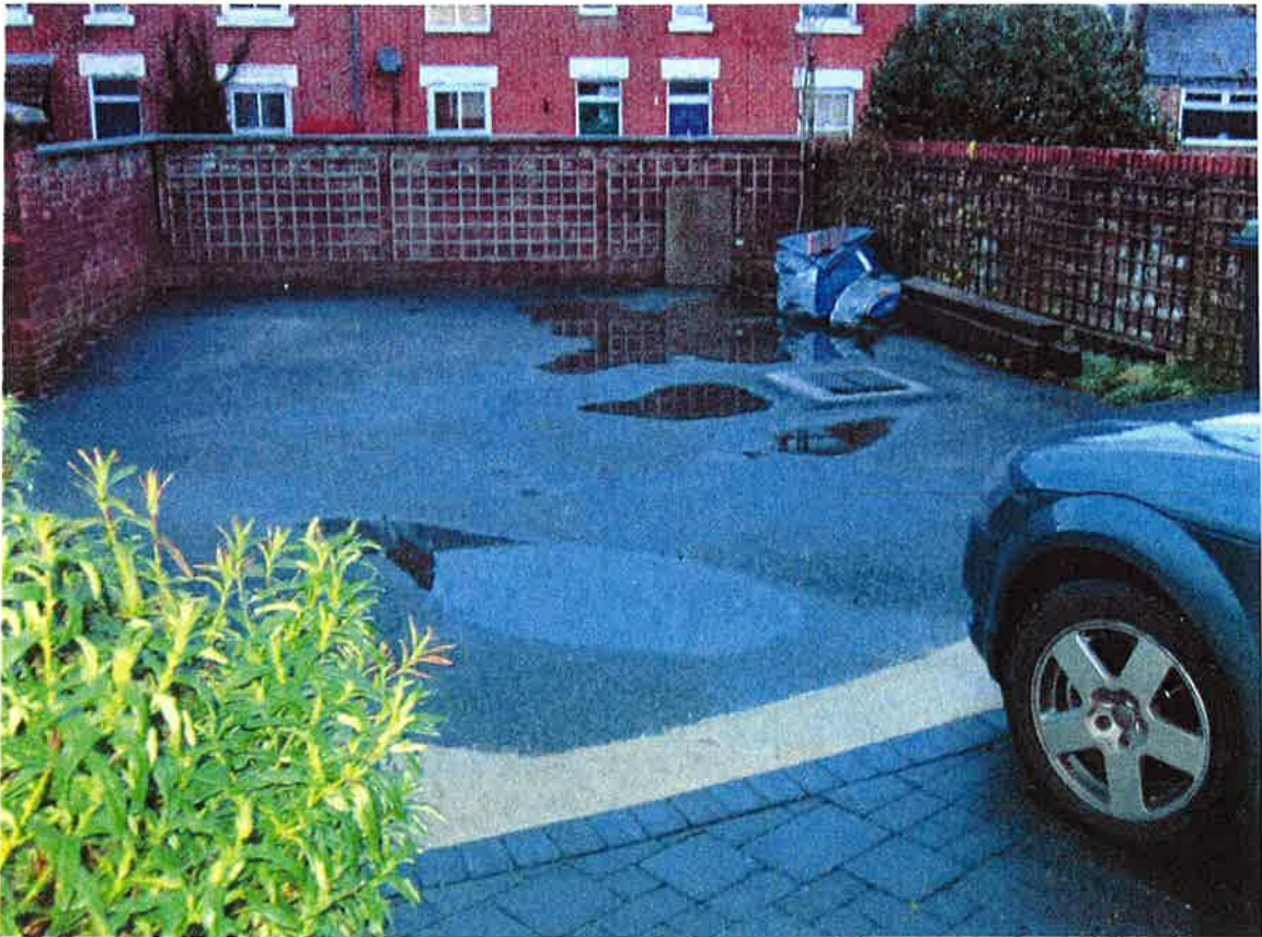
Puddles in Courtyard at No 78 Lower Rd.
